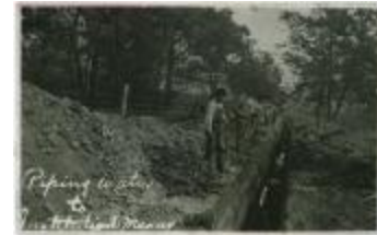
Students digging trenches for water pipes at the Mount Elgin Indian Industrial Institute, Muncey (13d-c5715-d23)
